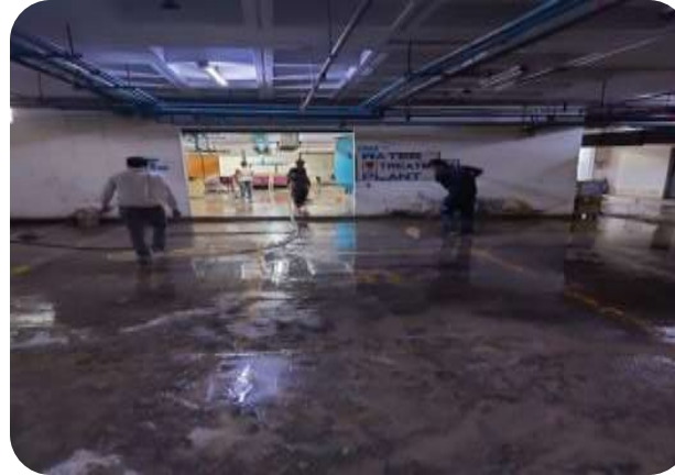
Reverse bleeding of grout from floor.
